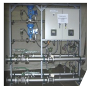
Water / Gas manifold
